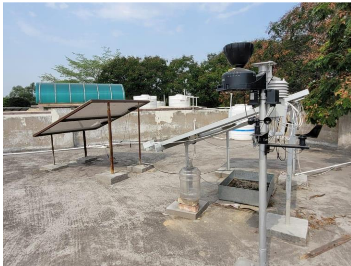
Rooftop 1 KW PV Panel installed in EEE Building
